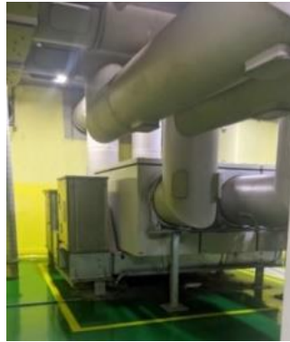
Gambar 2.20 Generator circuit breaker unit 3
