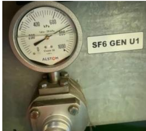
Gambar 4.2 indicator gas SF6 berkurang
