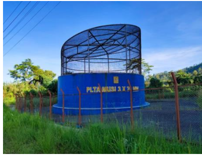
Gambar 2.3 Surge tank PLTA Musi
