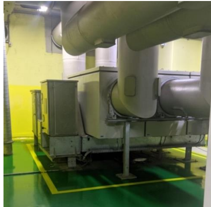
Gambar 4.1 Generator circuit breaker unit 3
